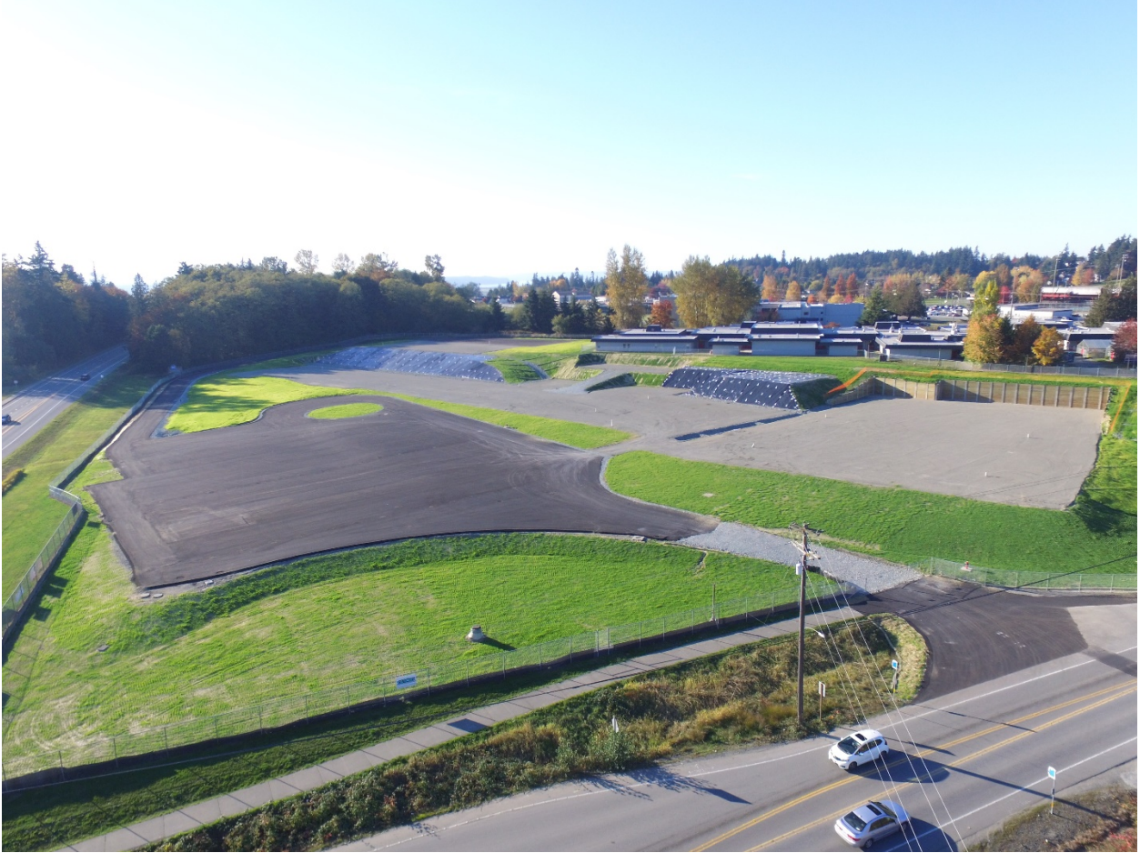
New SHS – Phase 1 – Site Prep Contractor: Taylor's Excavators June 2018 – November 2018 Aerial Photo taken by Kevin Cruse
